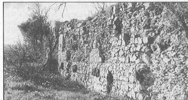
The Pisões dam: view from downstream, showing the partially preserved outside lining.
