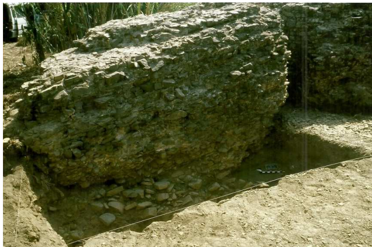
Figure 12. Dam of Álamo. Collapsed section of the dam. Photo J. L. Cardoso.
