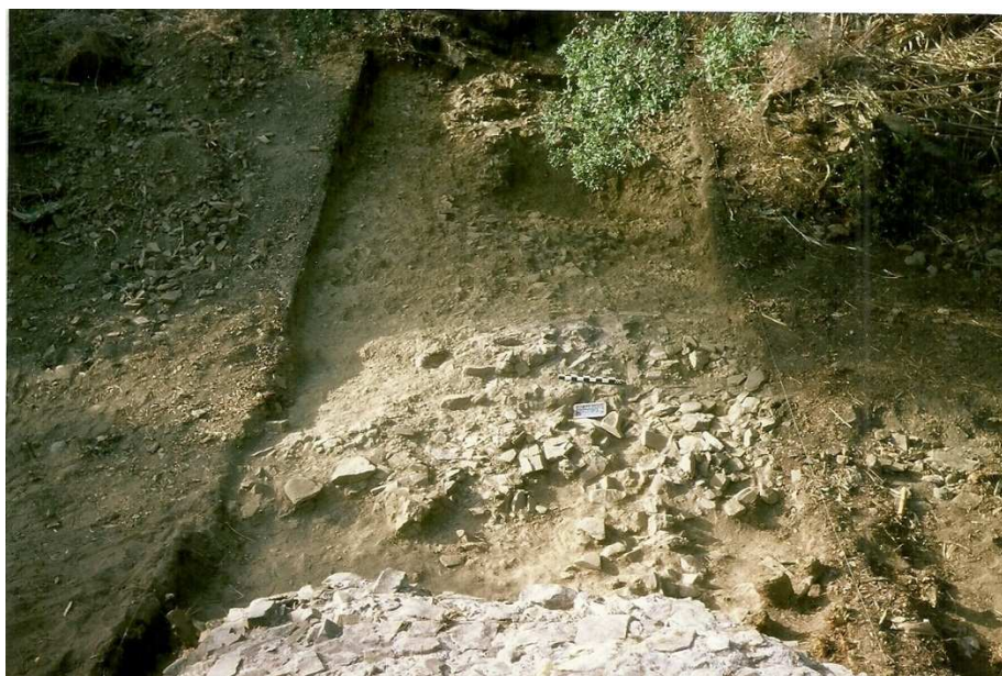
Figure 16. Dam of Álamo. Survey 2 (2006), evidencing the regularization of the geologic basement over which the dam was built. Note the remains of the foundation layer of the structure corresponding to blocks of greywacke cemented by a sandy-chalky mortar. Photo J. L. Cardoso
