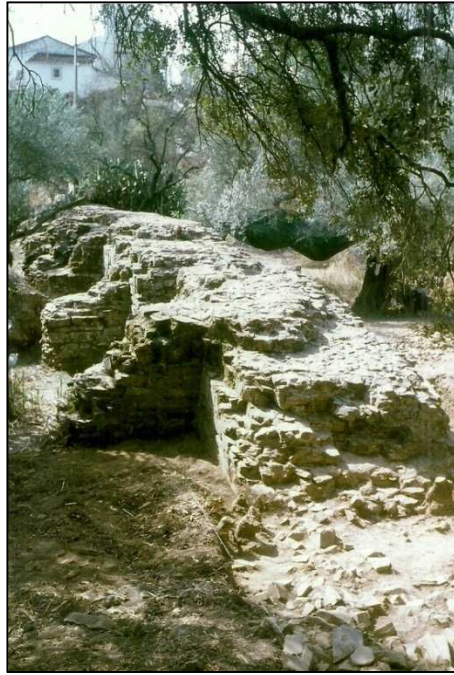
Figure 1. Dam of Álamo. General view. Note the constructive technique, by the successive layers of cemented blocks, that constitutes the nucleus of the structure. Both walls and buttresses are covered by horizontal layers of blocks of greywacke ( opus incertum ). Photo J. L. Cardoso.
