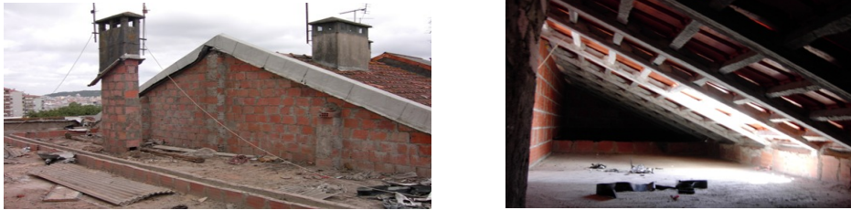
Figure 6. The interior and exterior view of the inclination of a gable roof.
