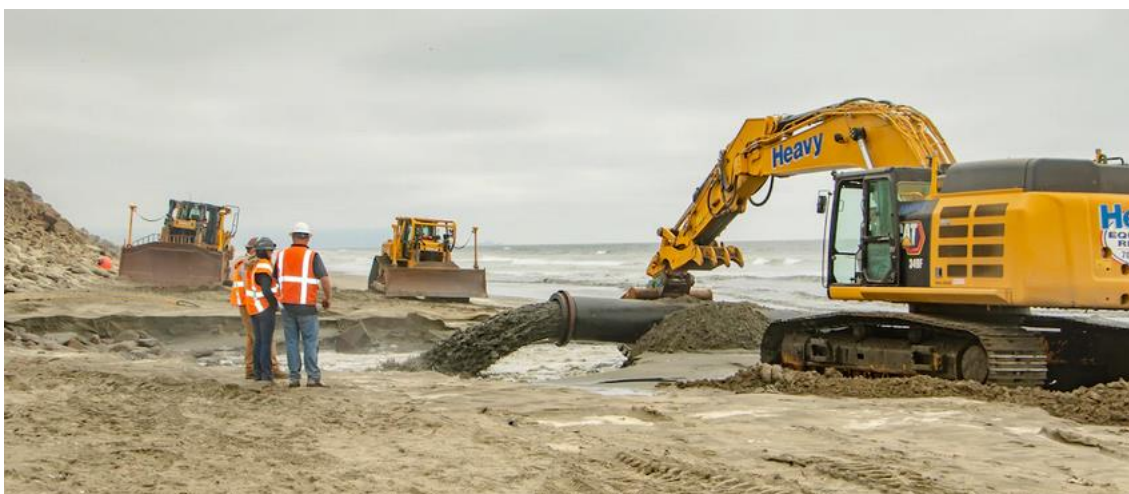
Figura 12 – Trabalhos de alimentação artificial de praia em Ocean Beach (San Francisco, Califórnia, EUA). Fonte: U.S. Army Corps of Engineers, San Francisco District Website – Public Domain – https://www.spn.usace.army.mil/Missions/Projects-and-Programs/Ocean-Beach-Beach-Nourishment/igphoto/2002848334/ .
